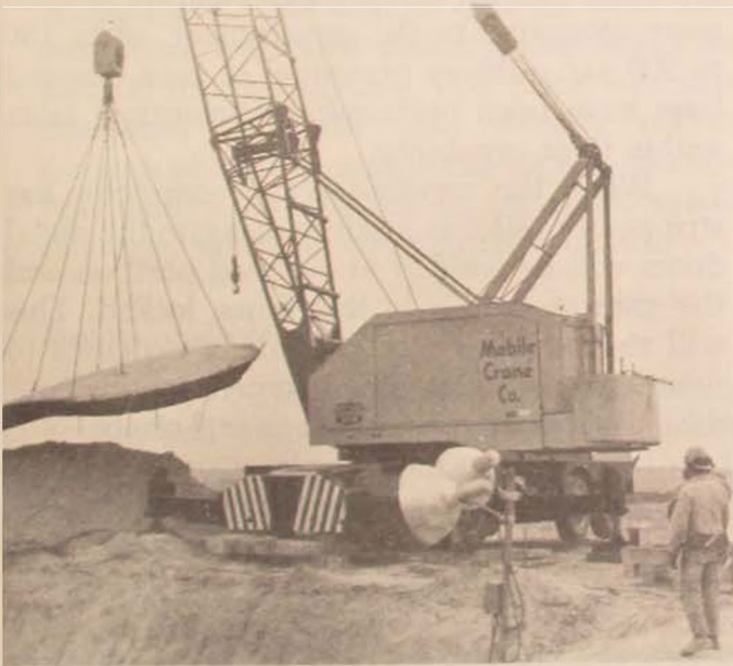
A 32-ton section of roof is lifted from the underground power plant.
